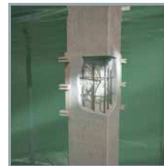
Conbextra UW has been specially formulated with anti-wash out agents for work in flowing water and tidal zones.
